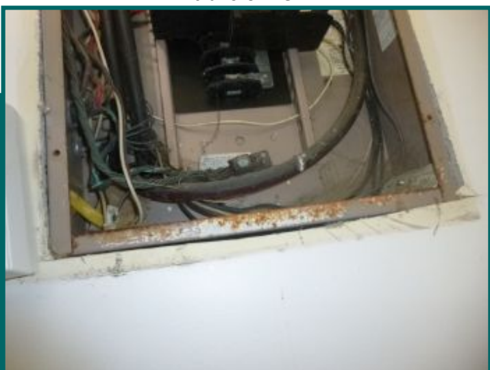
Corrosion at bottom of panel.
