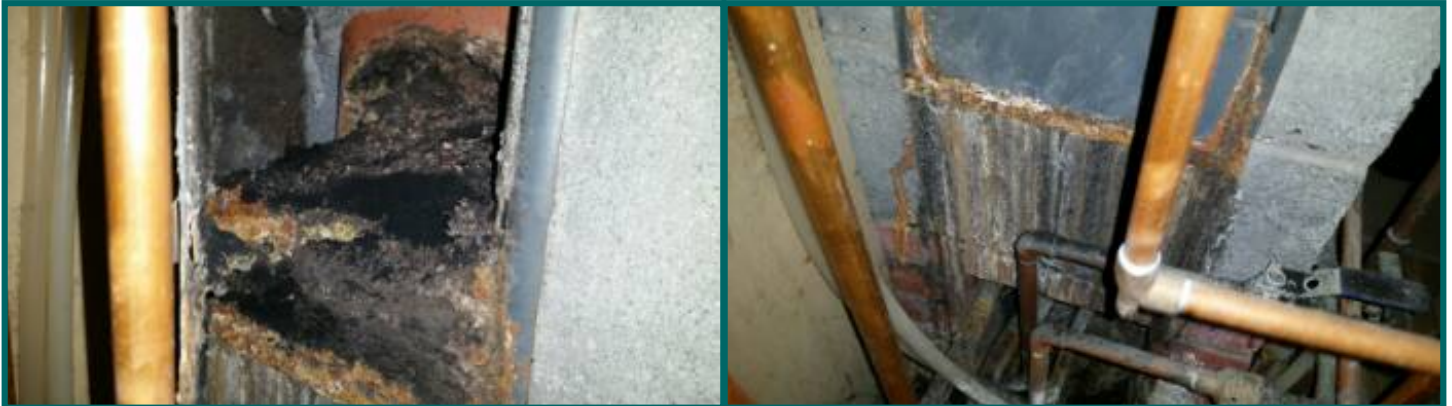
Chimney clean out
