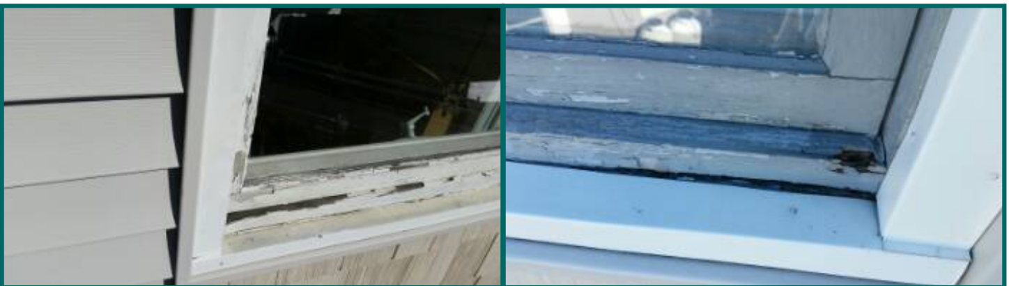
peeling paint at upper exterior window
