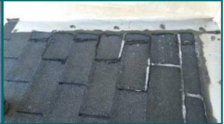
damage and prior repair to shingles over rear shed
