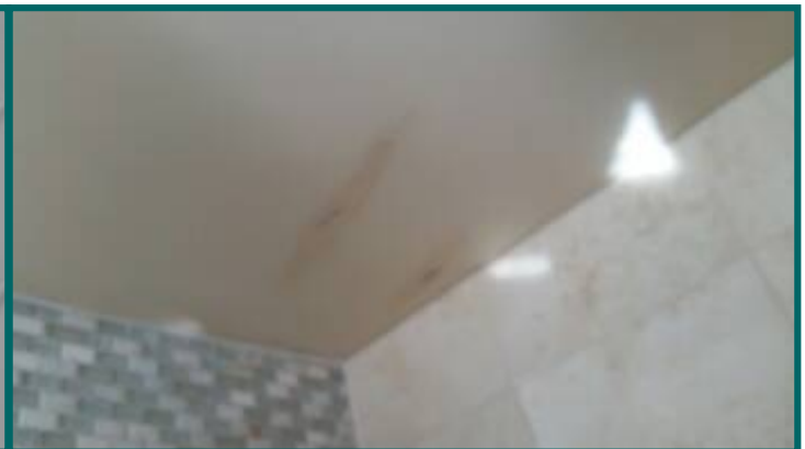
staining above shower
