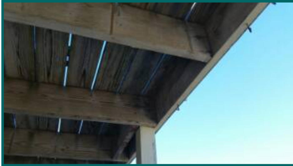
Missing Joist hangers.
