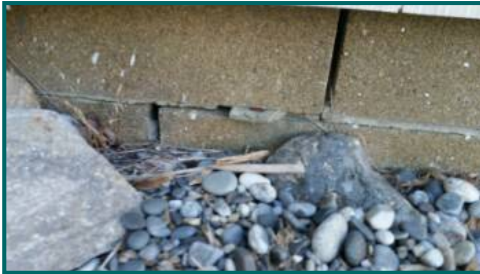
damage grout lines on left side of house
