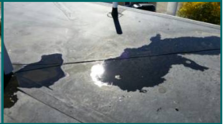
ponding on second upper room
