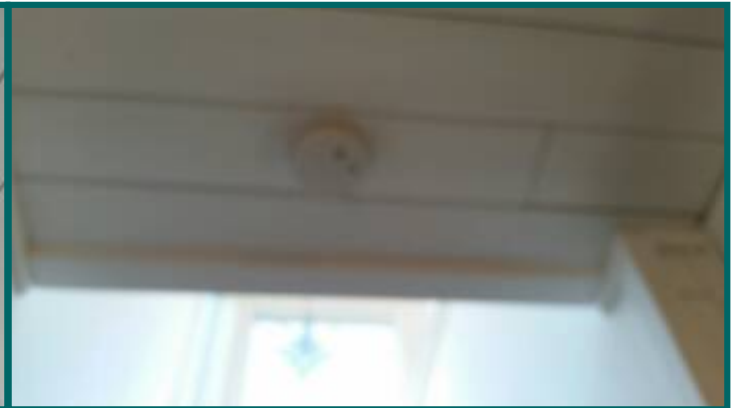
There is one smoke detector in bedroom hallway area, no smoke or CO detectors in bedrooms.
