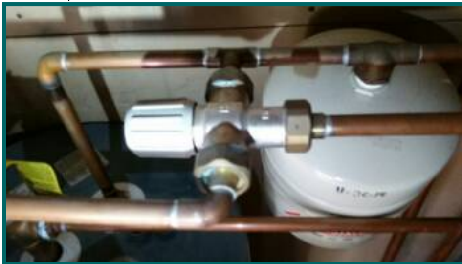
Mixing valve / burner control to adjust water temperature.
