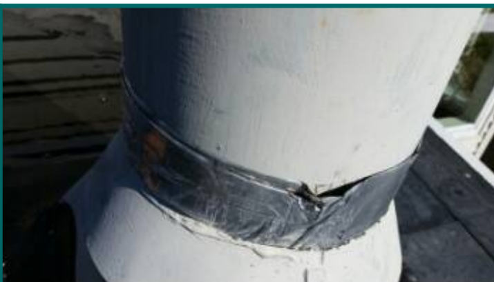
flashing tape is lifting on fireplace vent stack
