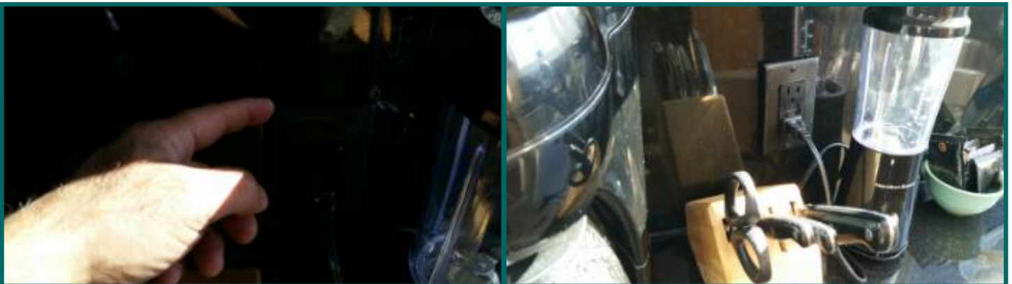
kitchen counter outlet is loose
