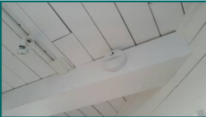
basement Hall has CO detector
