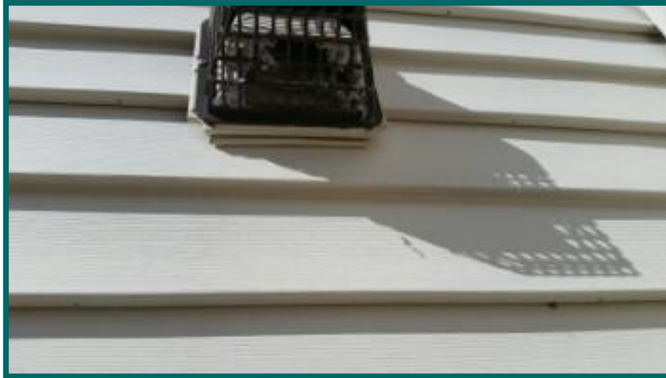
Dryer vent termination
