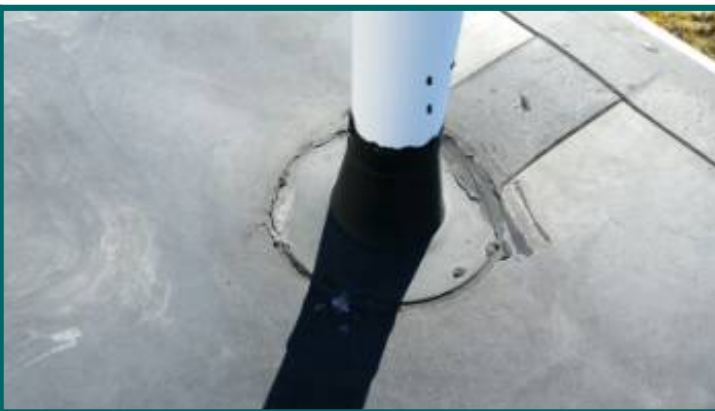
lower roof vent stack
