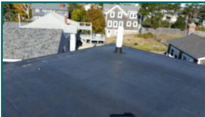
upper plumbing vent stack
