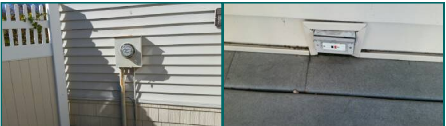
no power missing weatherproof cover at lower sliding door area
