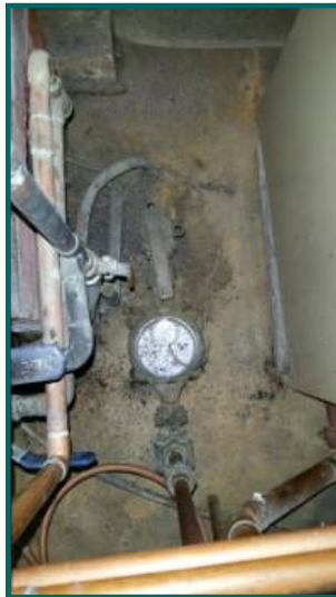
Main water shut off valve is located at water meter.
