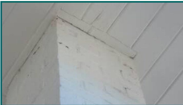
Ceiling stains at chimney roof penetration.
