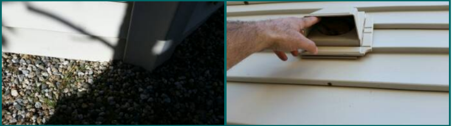
vent on left side of house is blocked with insulation
