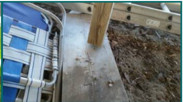
center post has no contact with ground or footing
