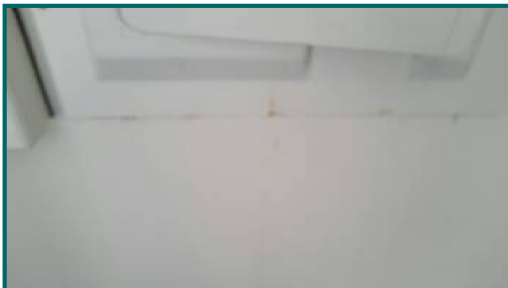
Staining below wall and bottom of panel
