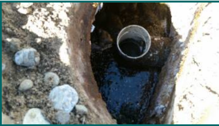
Septic tank outlet baffle.
