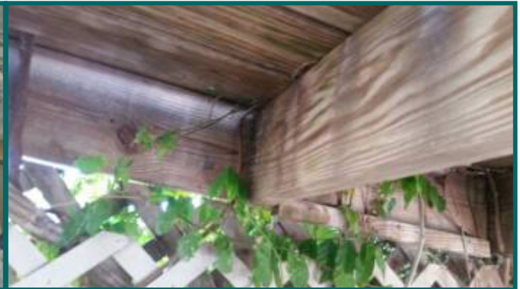
missing joist hangers at outside rim frame
