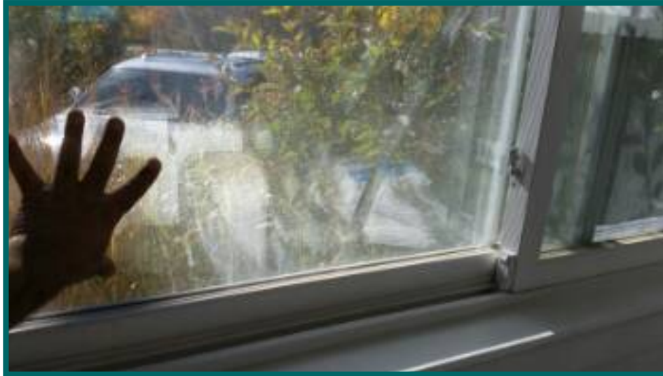
fogged window in basement bedroom
